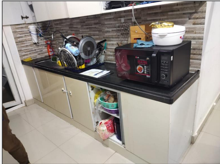
Discoloration of Laminate
